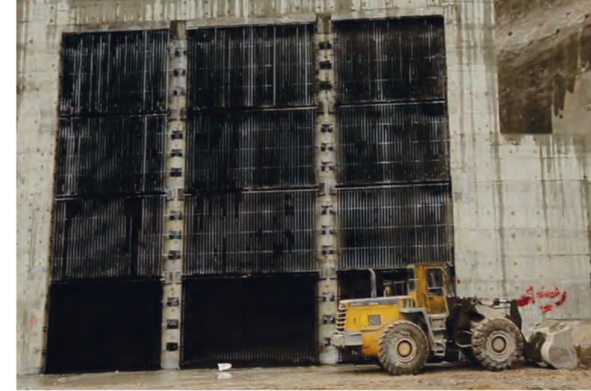
Trashrack 17x13 m, Rudbar lorestan Pumped Storage Power Plant
