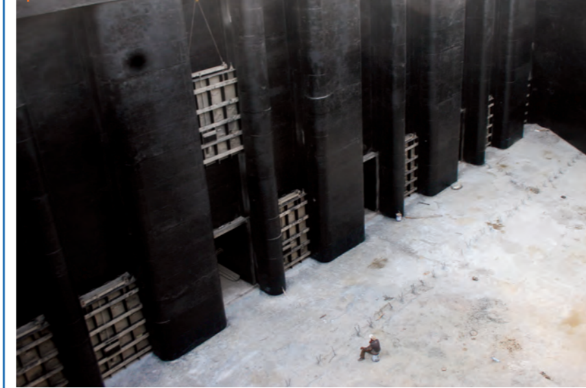
Stoplogs of water intake, persian gulf oil star refinery, Bandarabbas
